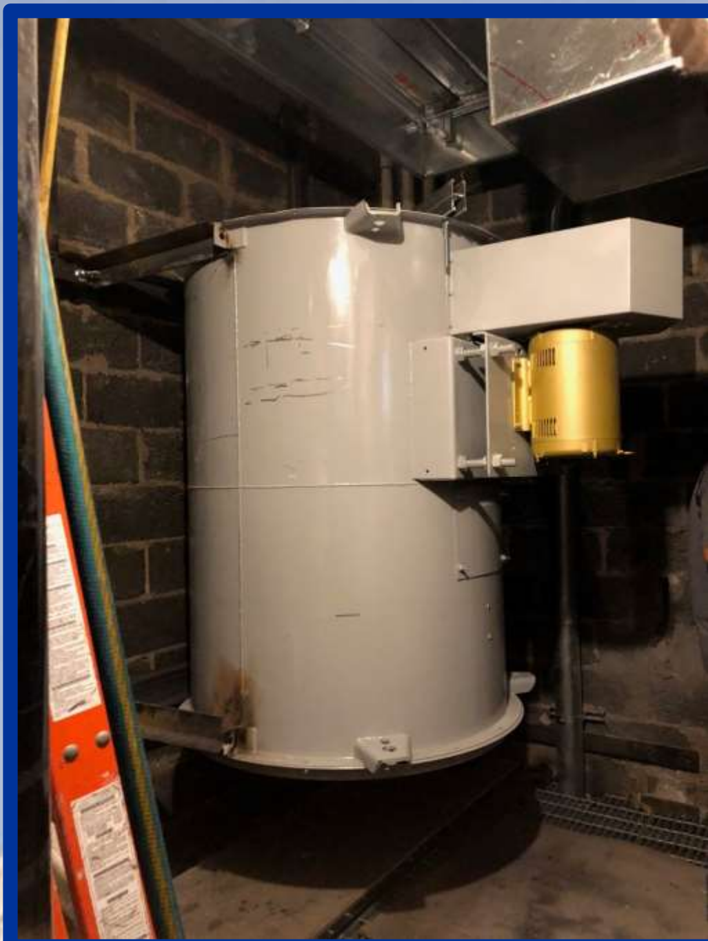
Return fans located within repurposed elevator shaftway conserves shaft space and maximized HVAC efficiencies.
