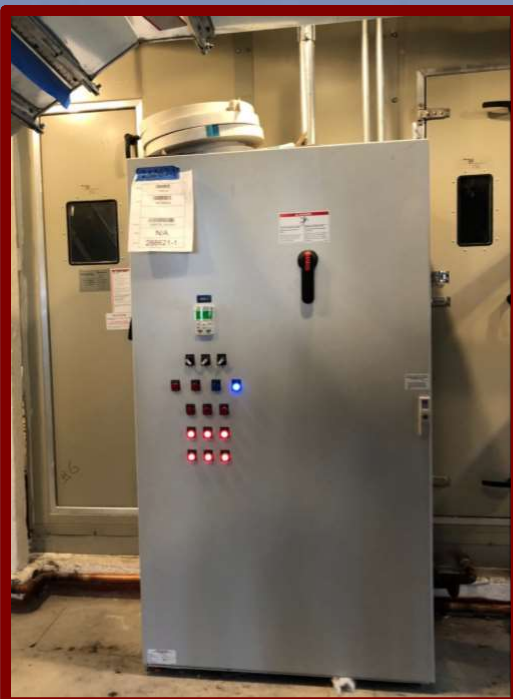
New Economizer Air Handling Units serve multi-floor tenants, and meet/exceeds NYC Energy Conservation Code (NYCECC).
