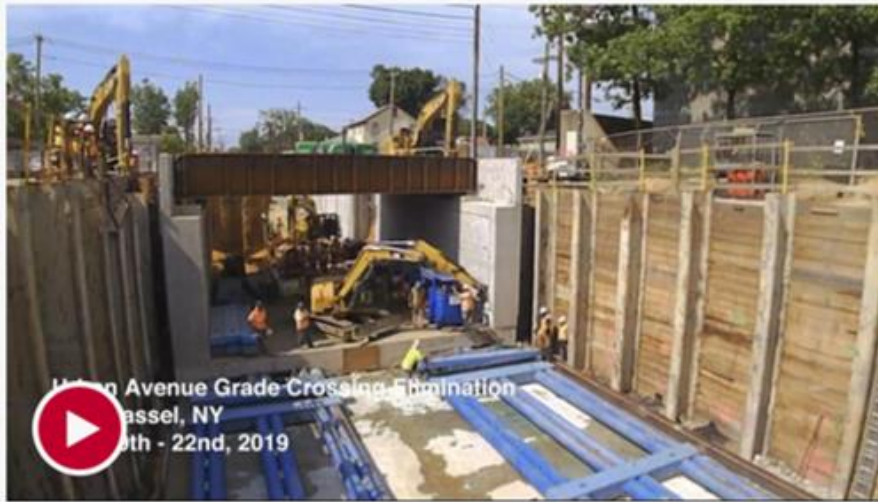
The LIRR on Thursday unveiled a new roadway underpass to replace a once-dangerous LIRR grade crossing on Urban Avenue in New Cassel, six months after construction began. Watch a time lapse of the work. Credit: MTA
