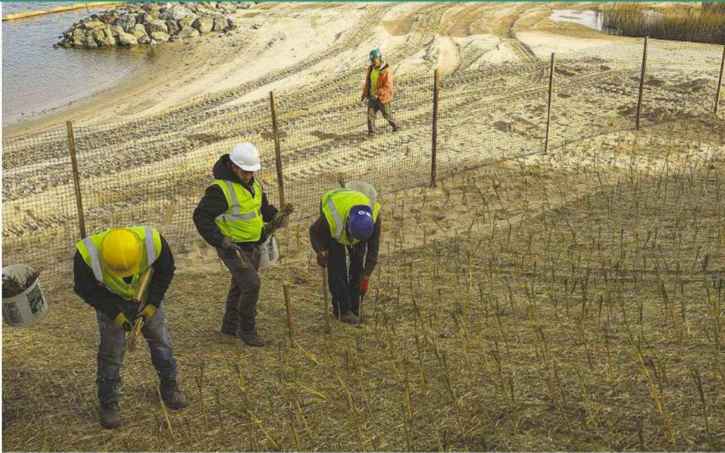
Workers place beach grass seedlings at the living shoreline project at Indian Island in Riverhead.
