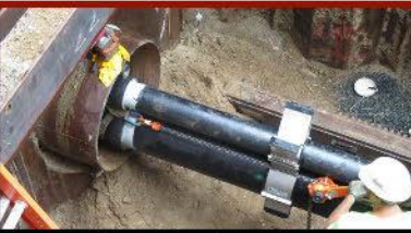
Ronkonkoma Hub Pump Station
