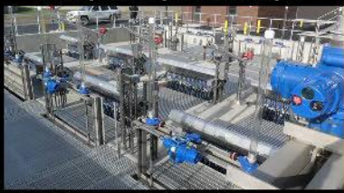
Bergen Point WWTP
