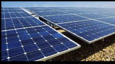
Smithtown Solar Photovoltaics
