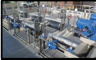
Bergen Point WWTP
