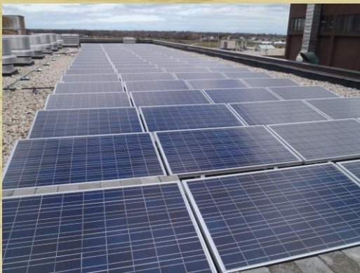
24-KW PV System Array
